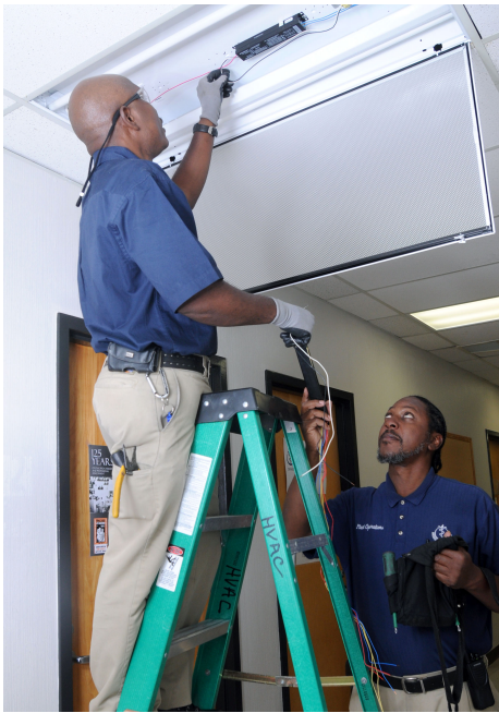
MSM UPGRADED 647 FLUORESCENT LIGHT FIXTURES WITH NEW, ENERGY-EFFICIENT BULBS AND BALLASTS TO SAVE OVER $16,000 IN ELECTRICITY COSTS PER YEAR.
